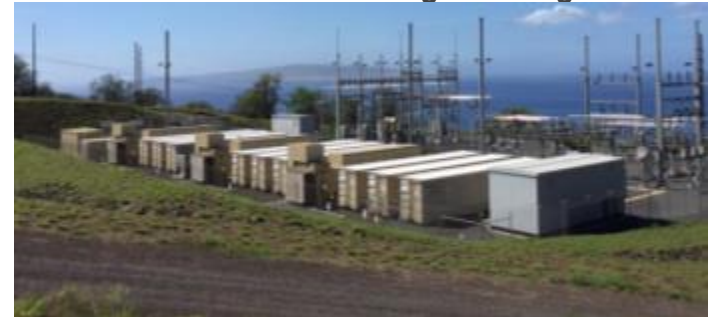
Standard containerized GSS ® grid storage solution
