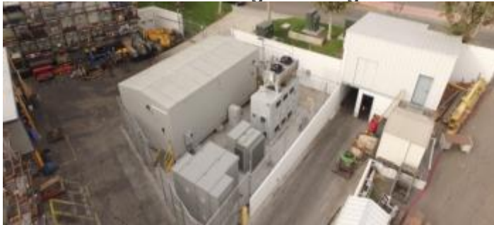
Custom enclosure GSS ® grid storage solution
